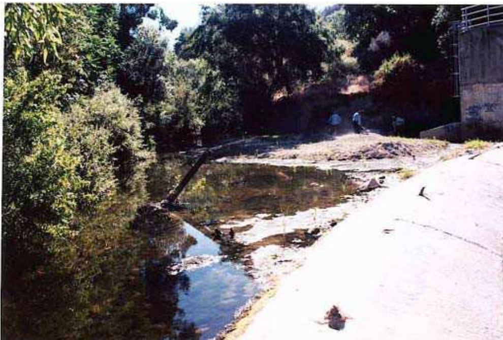
Excavation work for the low-flow stream inlet structures at the “slime slide”
