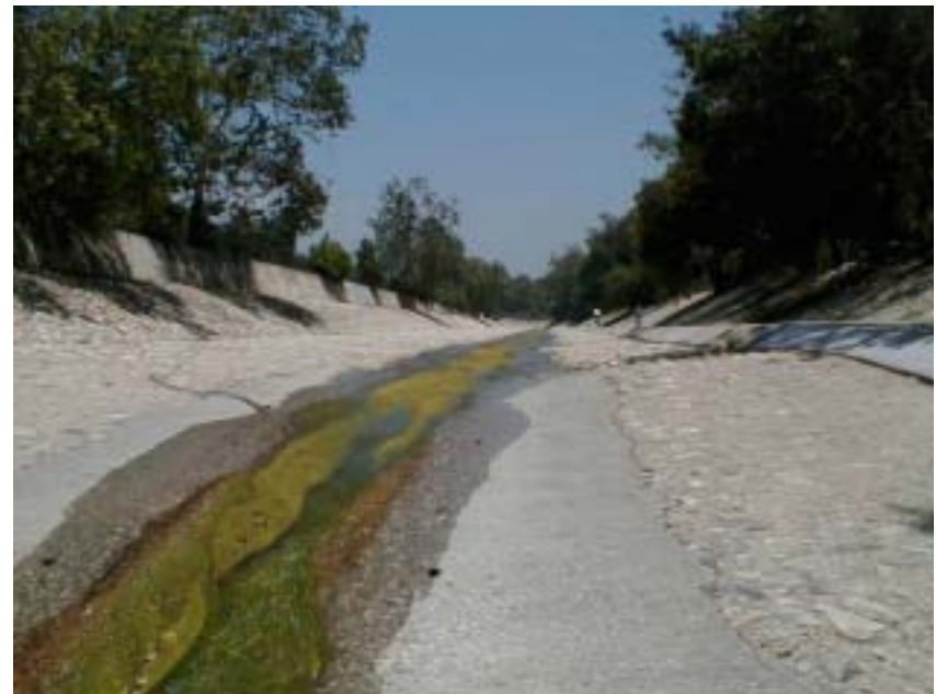
Polluted run-off water within the channel
