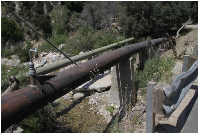
PWP's Diversion Pipeline
